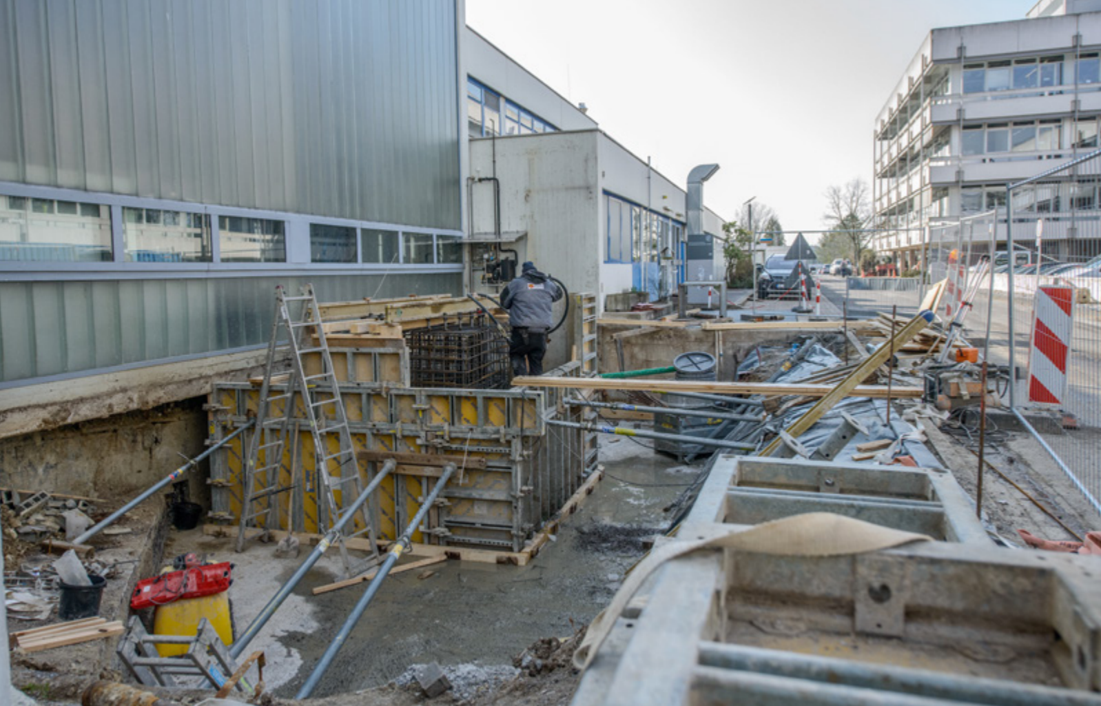
Baugrube vor der Energiezentrale Mitte Februar. / Excavation in front of the energy center in mid-February. (Foto: ibg)
